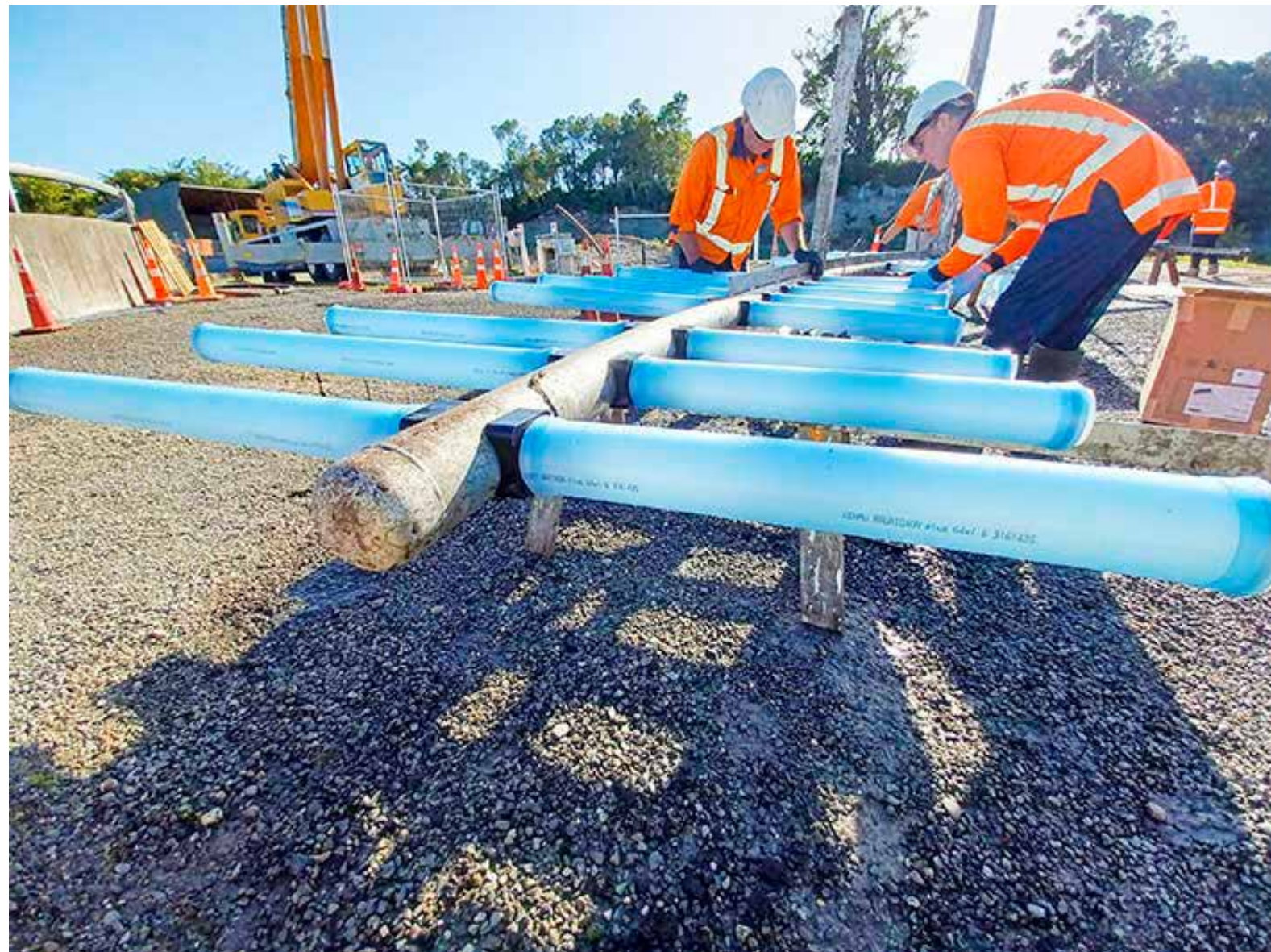
Above: Westport wastewater treatment plant diffuser assembly.
